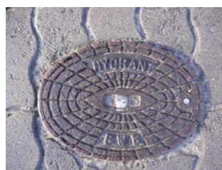
Slika 17: Oberfluthydrant, Vir: Lasten
